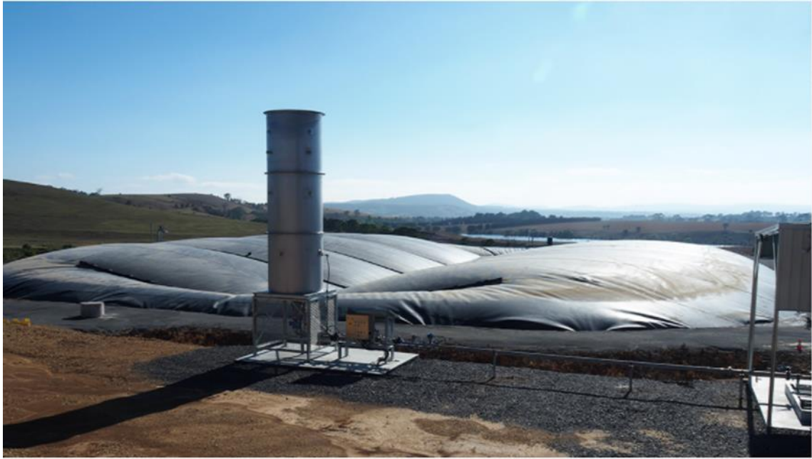
Figure 2: Hydroflux operated biogas plant
