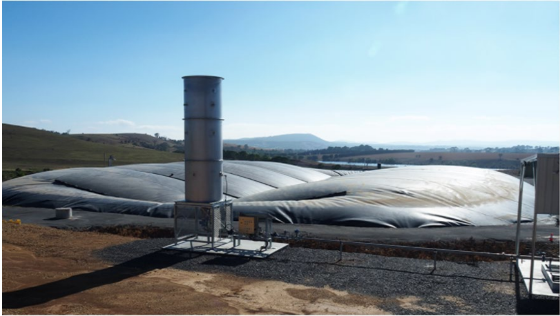
Figure 2: Hydroflux operated biogas plant
